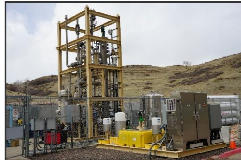
Biomethanation reactor (NREL)
